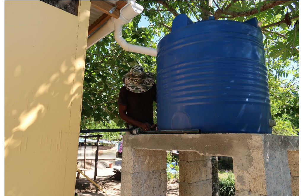
Rainwater tank for handwashing basins
