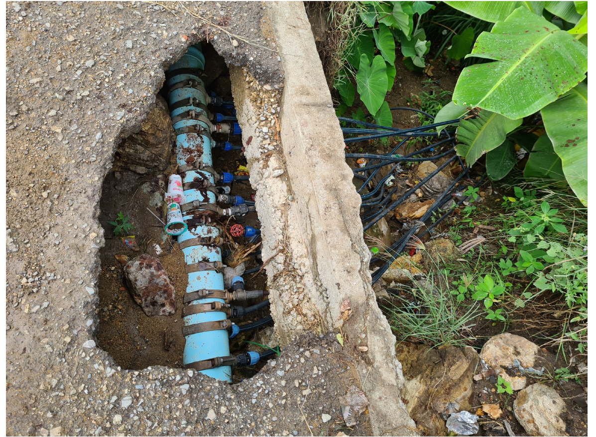
16 x Illegal connections to the Water PNG Distribution main on Pari Road (June 2022)
