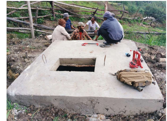
Water infrastructure: Reservoir tank
