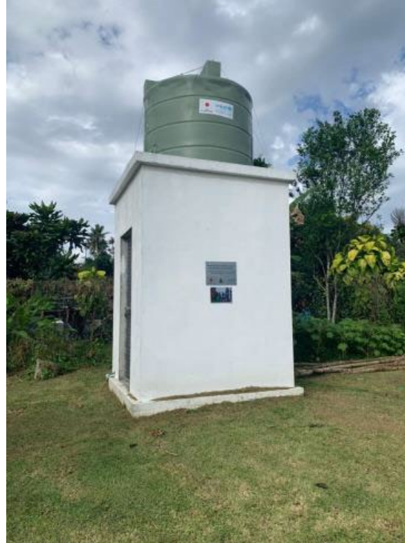
Indirect Gravity Fed System Tank stand built as a concrete kiosk to accommodate solar panel control unit against severe weather at Mele Health center.
