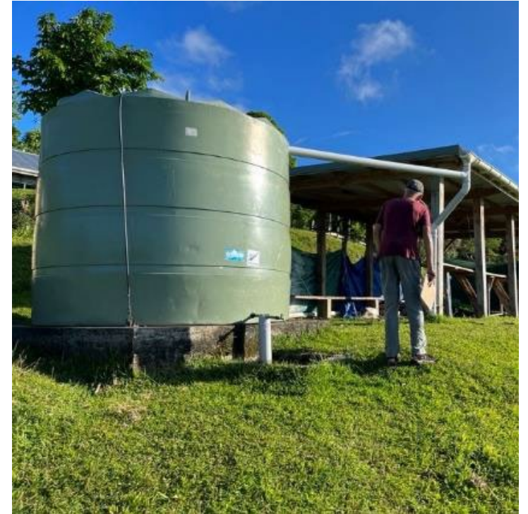
Rainwater Harvesting System built with cyclone straps.
