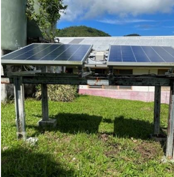
Solar Panels are installed in a way that's easy to dismantle before a cyclone hits
