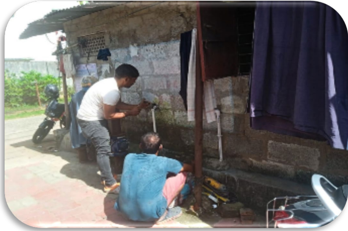
Household pipeline connection
